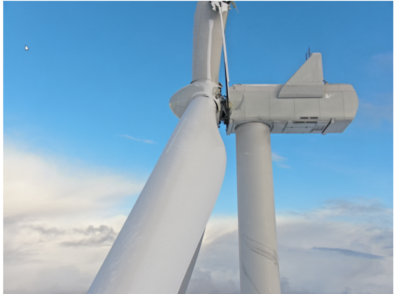
Significant blade, nacelle, hub and possible tower damage
